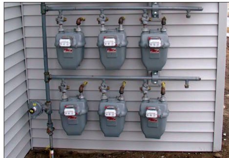
Figure 2 – A meter bank allows meters to be placed on a sidewall and hidden from the street. Meter banks can easily be hidden with landscaping or fencing to help offer more curb appeal.
